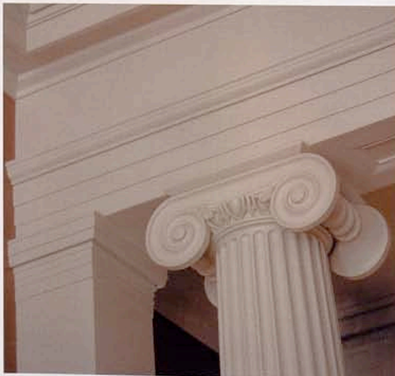
The proportions and detailing of the columns, anta pilasters and entablature of the Ionic column screen were derived from Minard LeFevre pattern books from the 1830s as well as from other period archaeological survey drawings from the Greek temple at Illisus. Three different craftspeople were involved in these columns: Visions in Plaster in New York City produced the drawn plaster moldings, Ahmad Suleiman made the anta and column capitals and Toronto, Ontario-based Balmer Architectural Mouldings custom made the turned plaster column shafts and bases.
